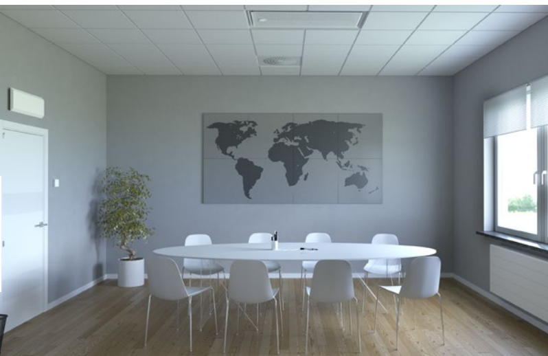
Conference room with setpoint selector switch and demand-controlled air regulation as well as waterborne cooling and control of radiators.
