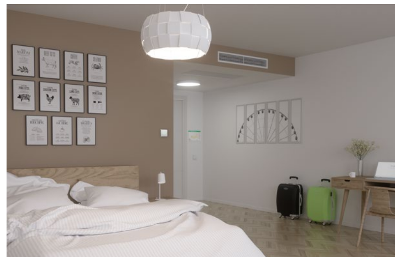
Hotel room with setpoint selector switch, waterborne cooling and heating as well as demand-controlled air regulation. Key card holder for occupancy.
